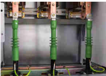
AIS20 with mechanical cable lug
