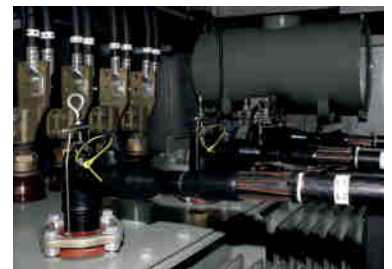
Transformer connection with 158LR
