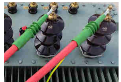
AIP20 as a transformer connection
