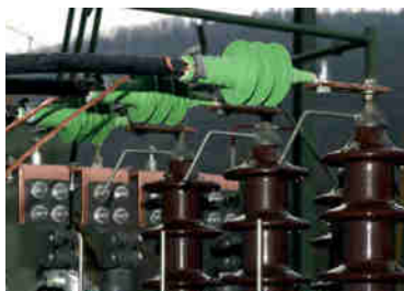
AFN10 as a transformer connection
