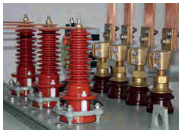
PITO-E on transformer with bushings
